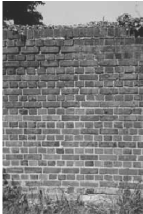
English Bond brick pattern: alternating courses of all stretchers and all headers
