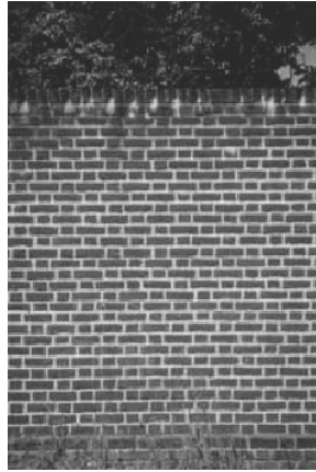
Flemish Bond brick pattern: every course consisting of alternating stretchers and headers
